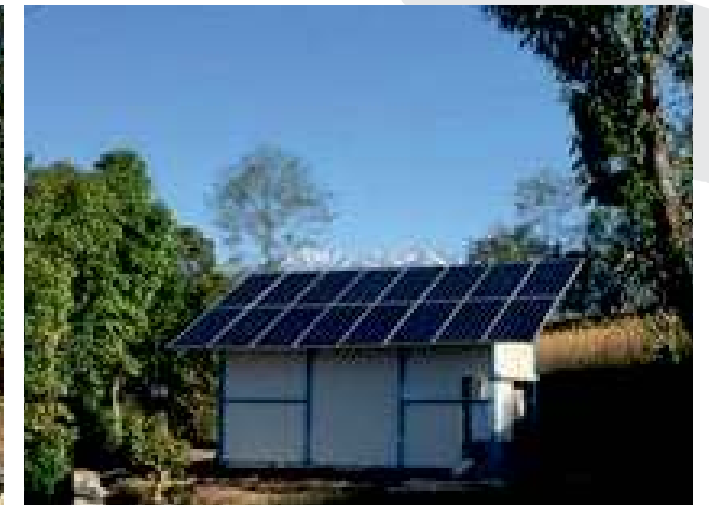
100% grid and diesel free: Powered by solar energy; net-zero carbon footprint.
